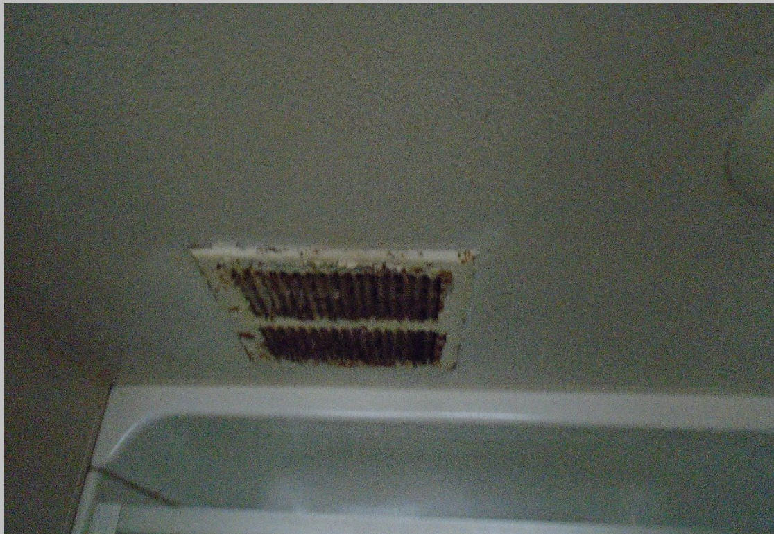
BIOLOGIC STAINING ON BATH EXHAUST
