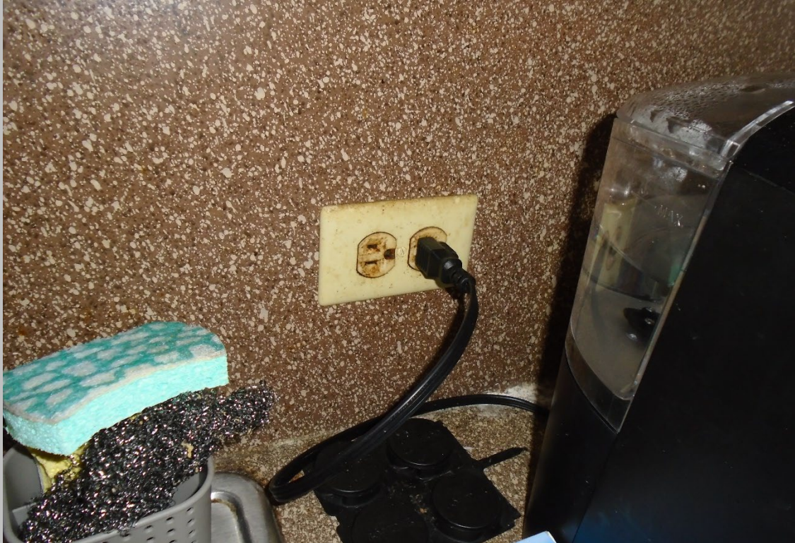
NO GFCI IN KITCHEN
