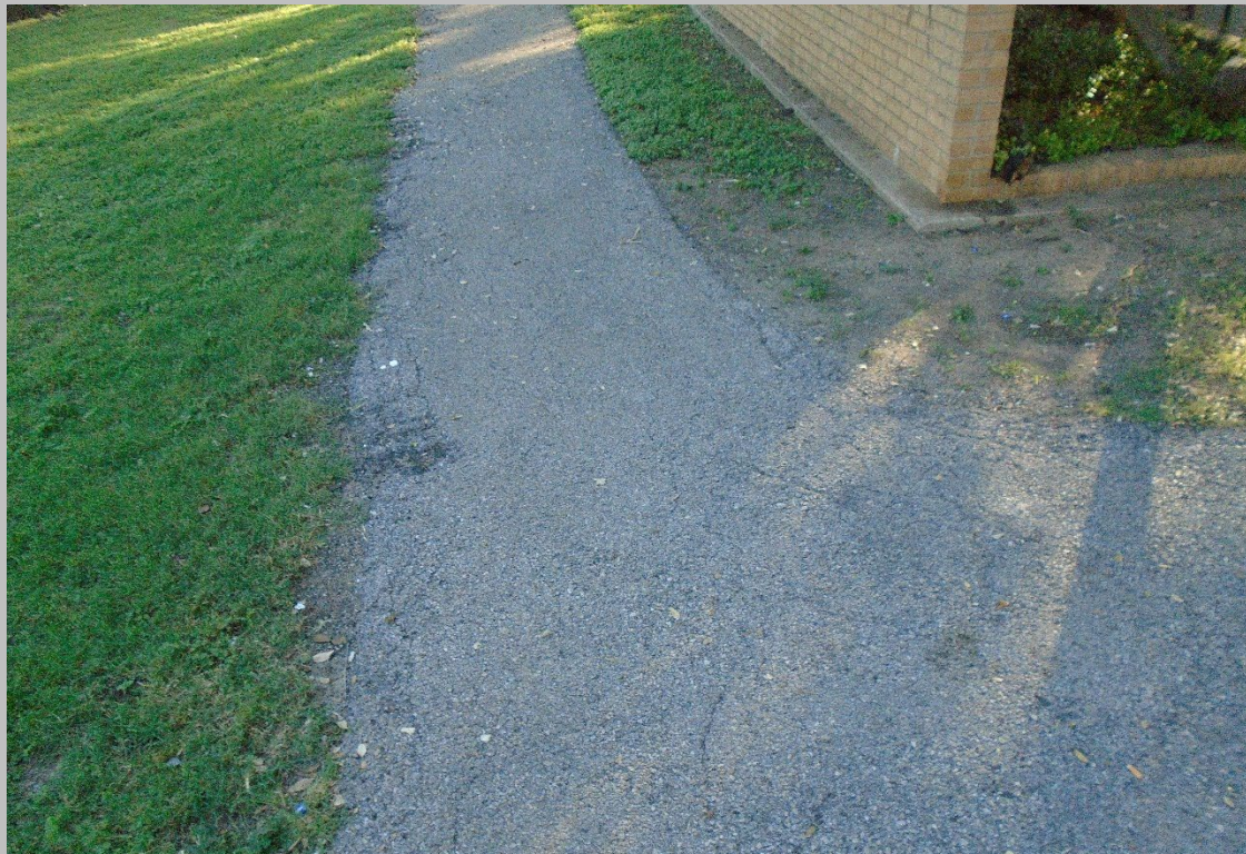
FLATWORK REPAIR NEEDS
