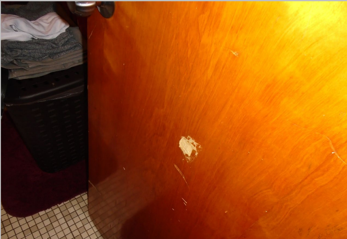
UNIT DOOR REPAIR NEEDS
