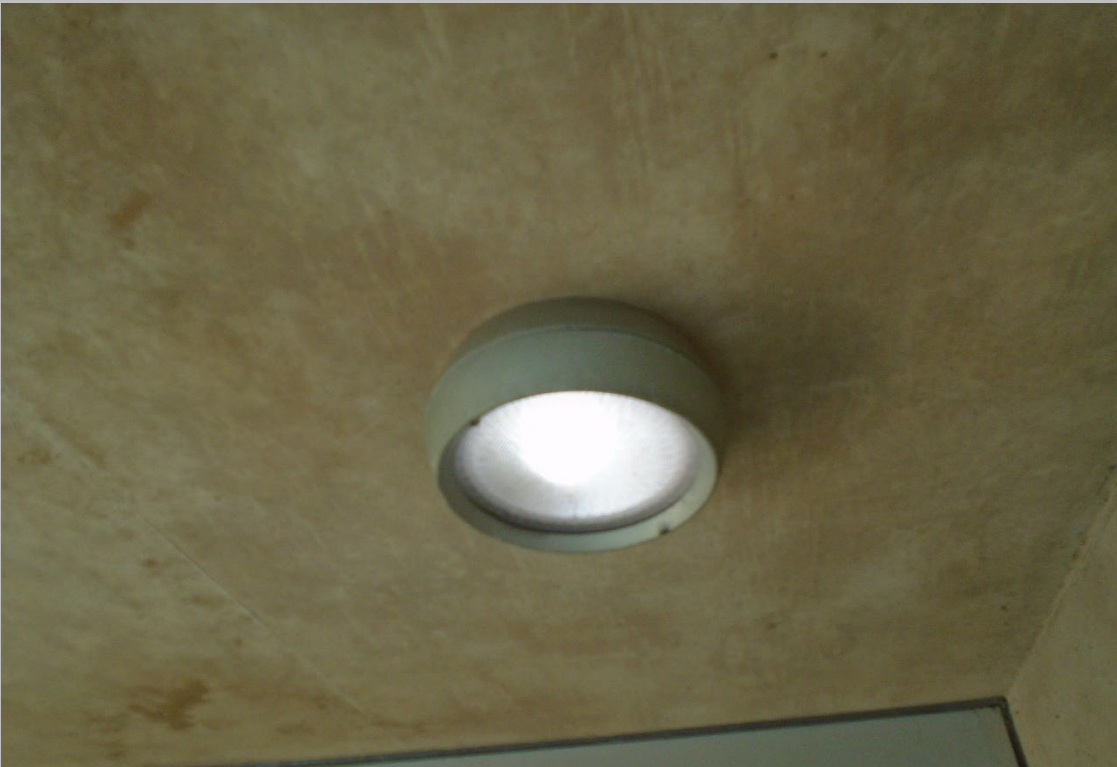
EXTERIOR LIGHTING REPAIR NEEDS
