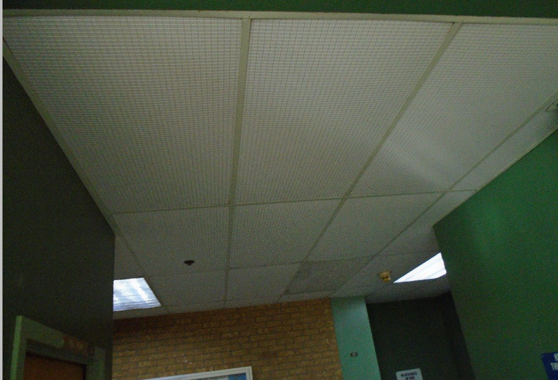
CEILING TILE REPAIR NEEDS
