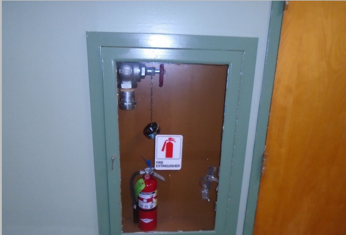
HOSE CABINET AND STANDPIPE OUTLET
