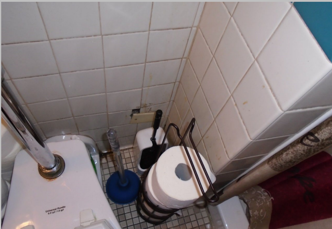
TILE REPAIR NEEDS
