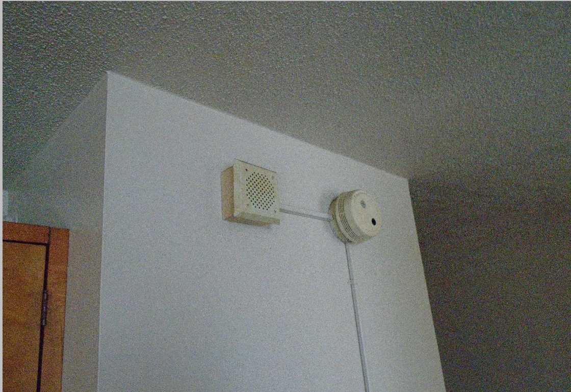
SMOKE DETECTION EQUIPMENT
