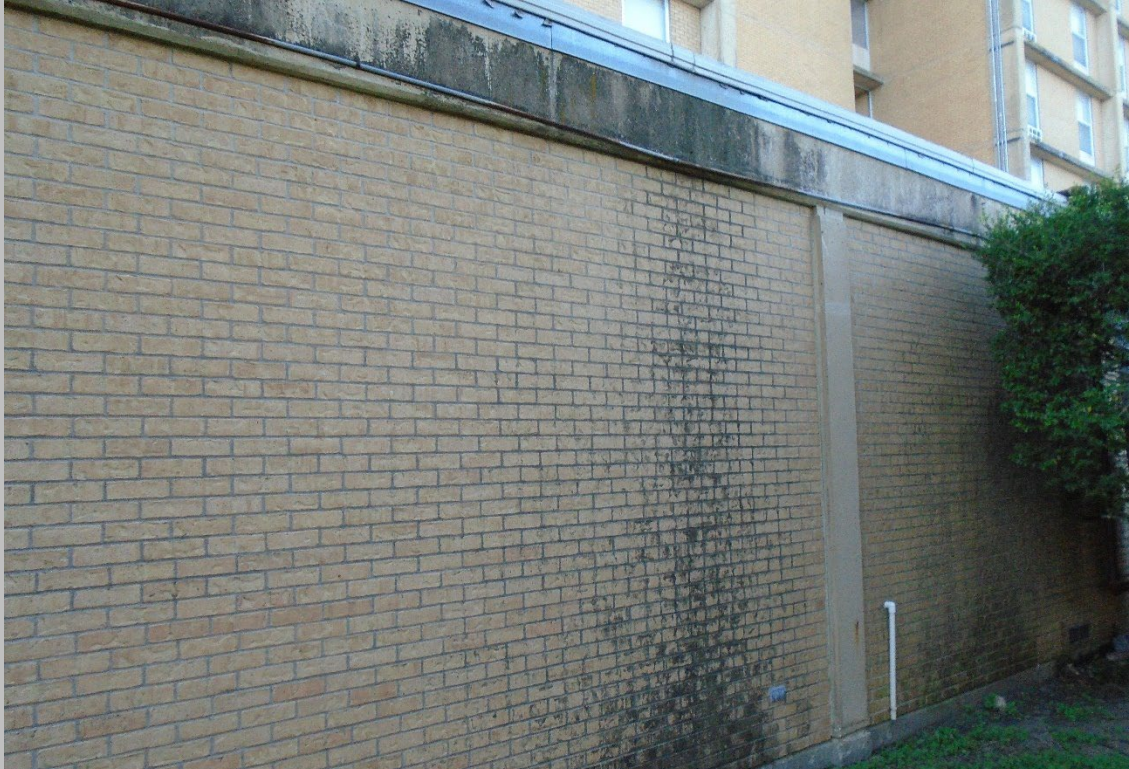
BIOLOGIC STAINING ON MASONRY
