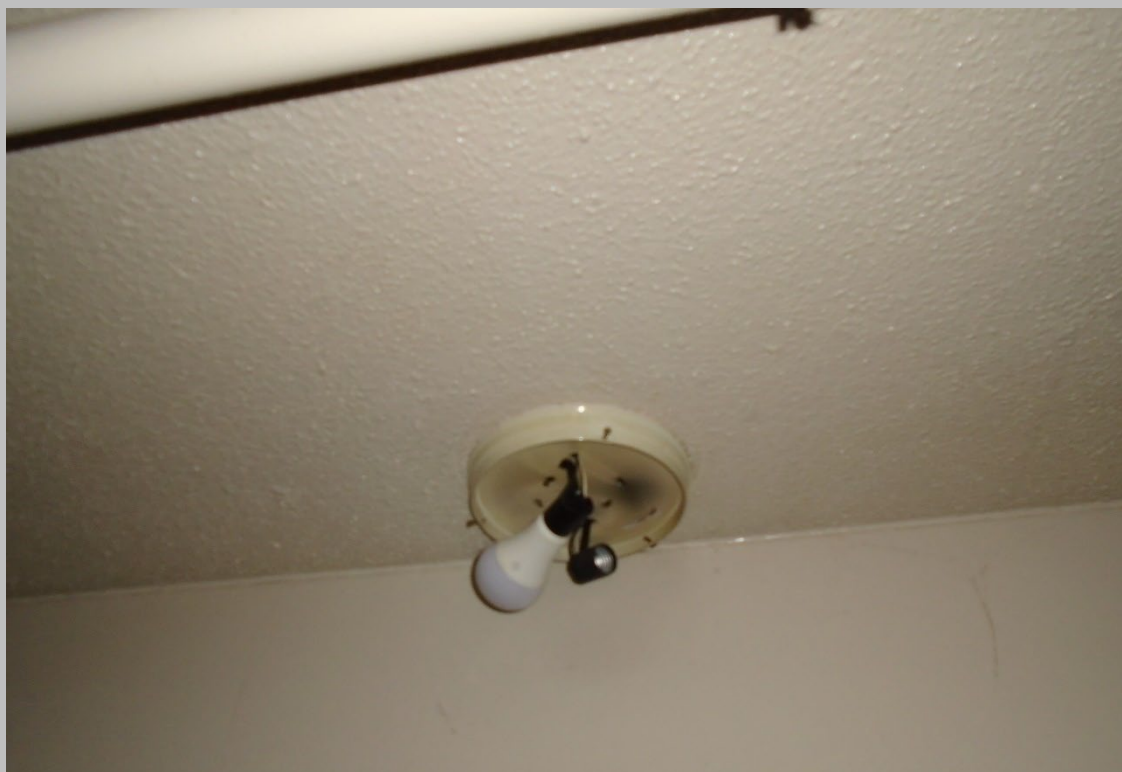
ISOLATED LIGHTING REPAIR NEEDS
