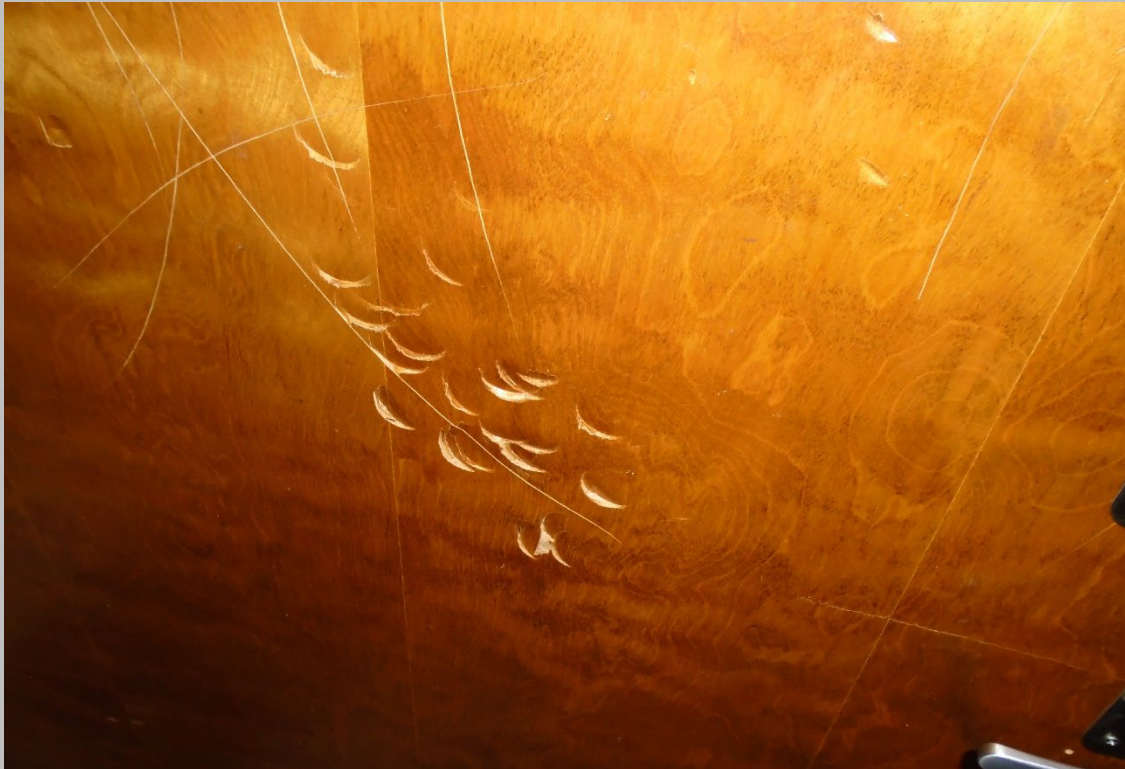
UNIT DOOR REPAIR NEEDS
