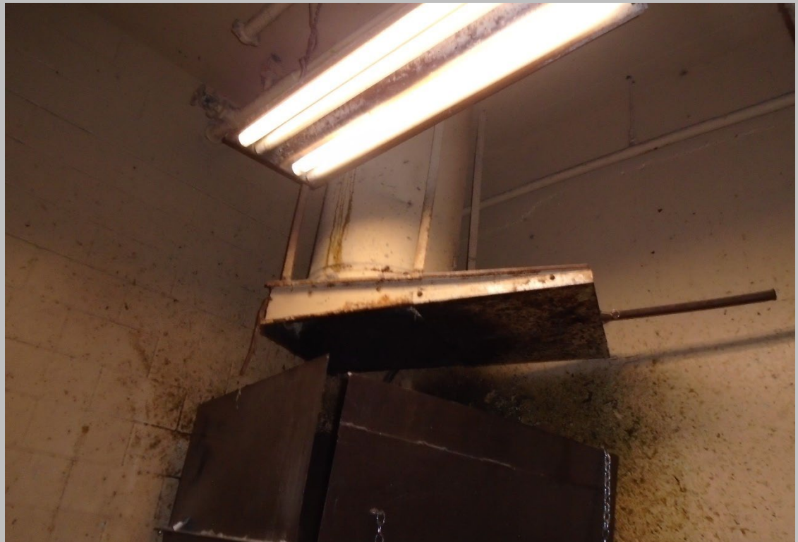
REFUSE CHUTE/ COMPACTOR
