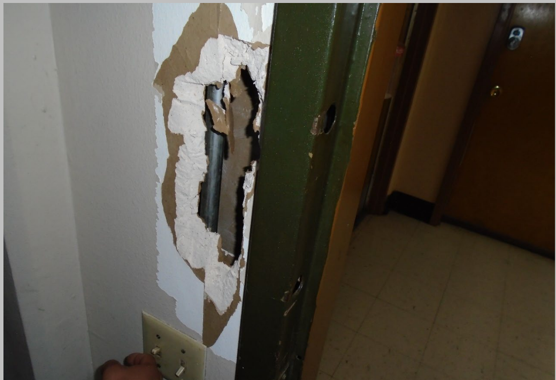
ISOLATED DRYWALL REPAIR NEEDS
