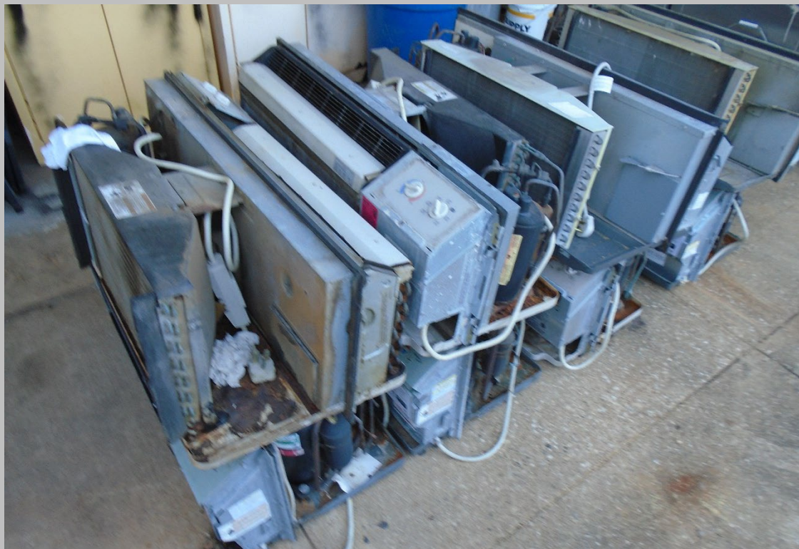
TYPICAL PTAC CONDITION
