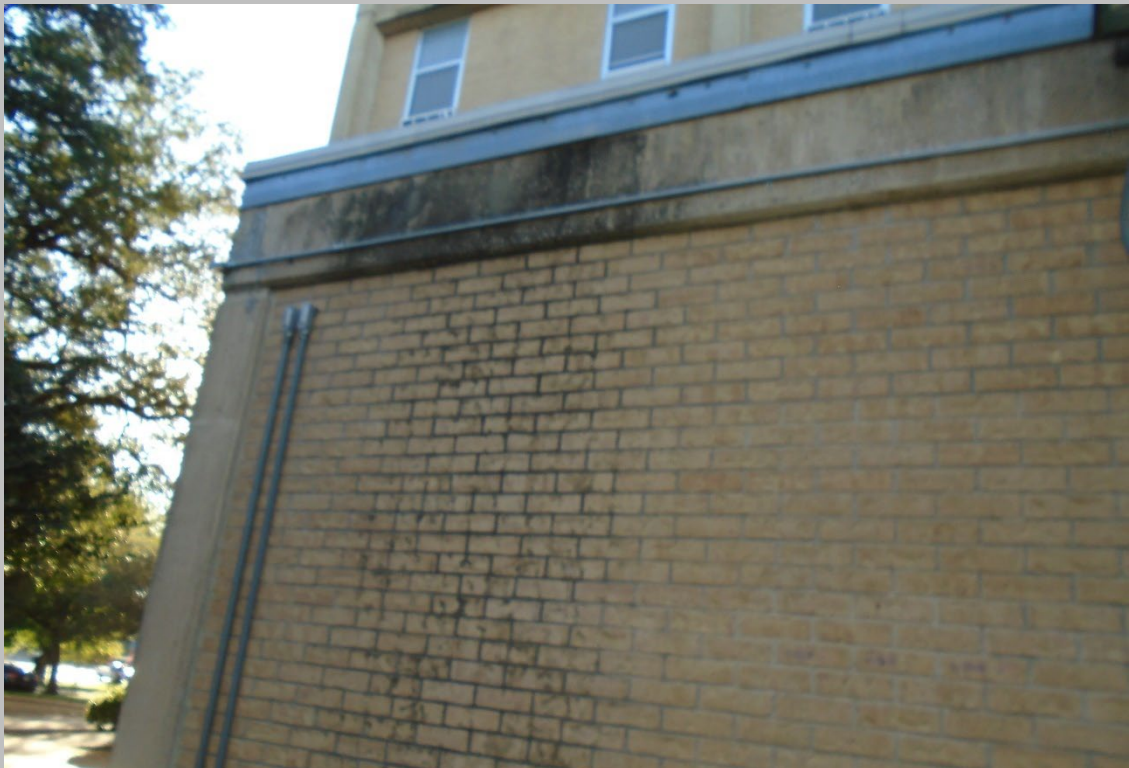
BIOLOGIC STAINING ON MASONRY
