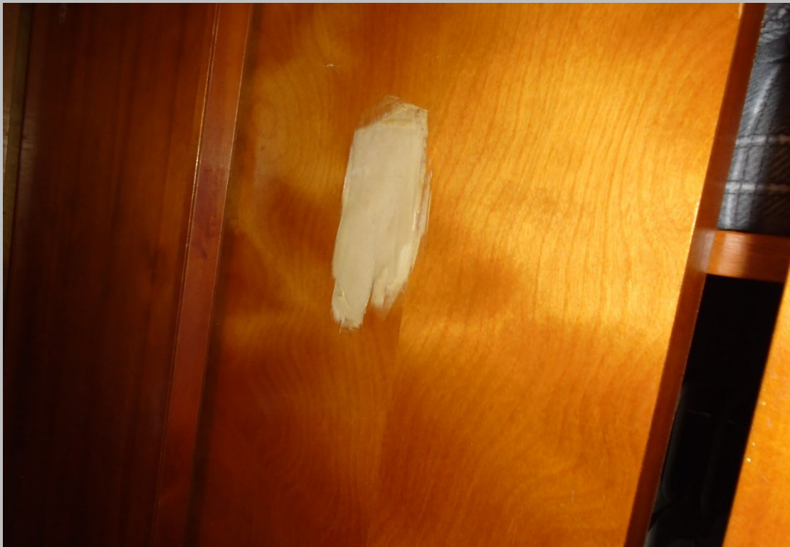
UNIT DOOR REPAIR NEEDS
