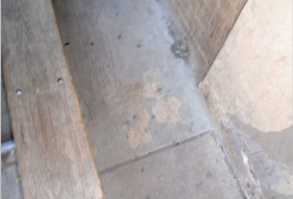
CONCRETE REPAIR NEEDS
