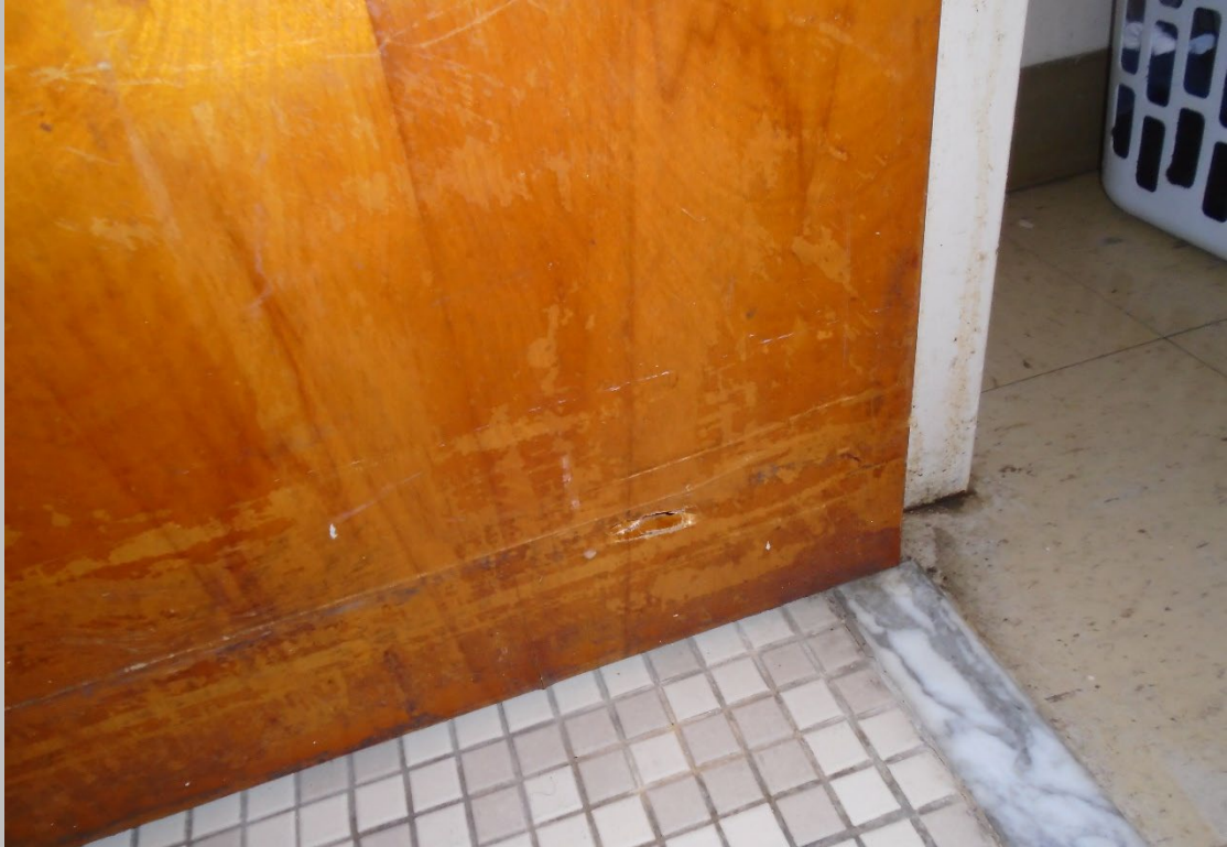
UNIT DOOR REPAIR NEEDS
